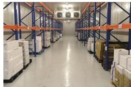
Figure 9: A typical cold room
