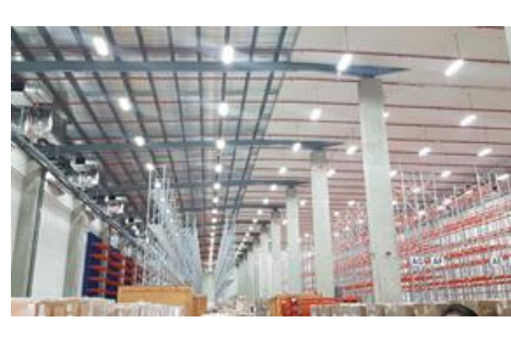
Figure 6: DHL's air-conditioned room
